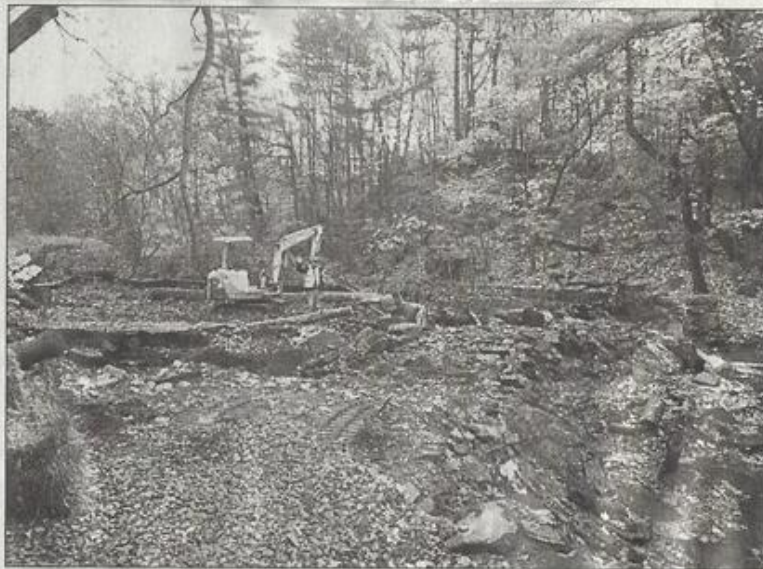
A photo of the sediment removal work underway. Photo courtesy of the Friends of Gorham's Pond.
